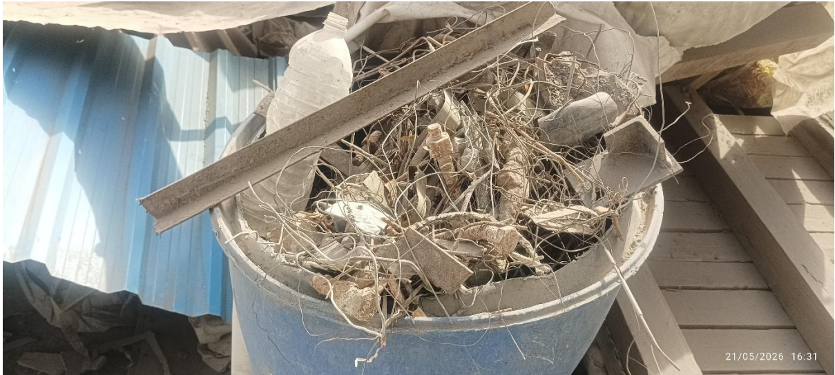
Cement attached mix steel
