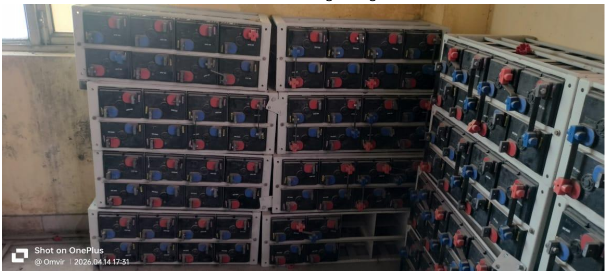
Scrap Battery 2V,240 AH MAKE EXIDE
