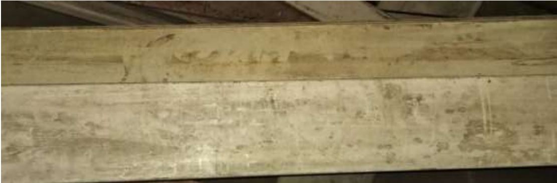
Electrical Aluminum cable
