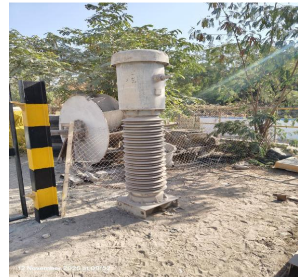
LOT 4 SCRAP CURRENT TRANSFORMER PIC3
