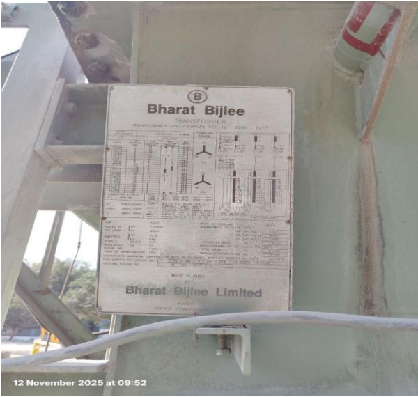
LOT 3 SCRAP POWER TRANSFORMER Part 2
