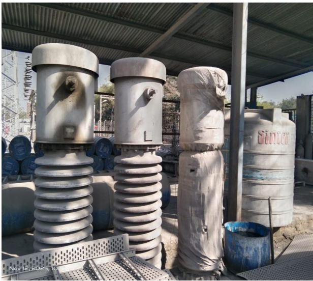
LOT 4 SCRAP CURRENT TRANSFORMER PIC1
