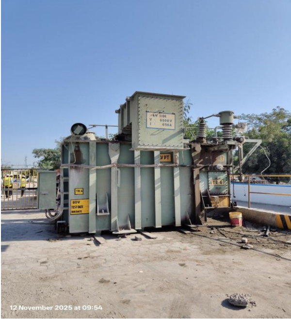
LOT 3 SCRAP POWER TRANSFORMER Part 1
