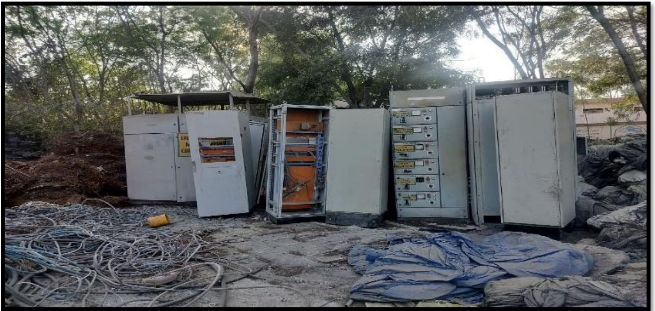
ELECTRICAL PANEL-USED-9 nos.
